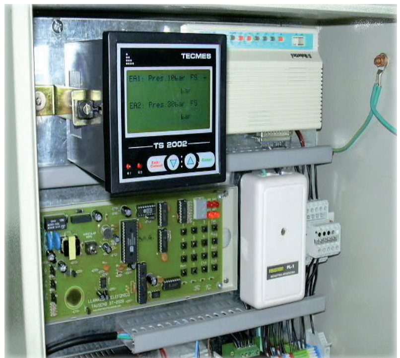
Pressure control in gas pipelines, Gas NEA, Entre Ríos, Argentina
