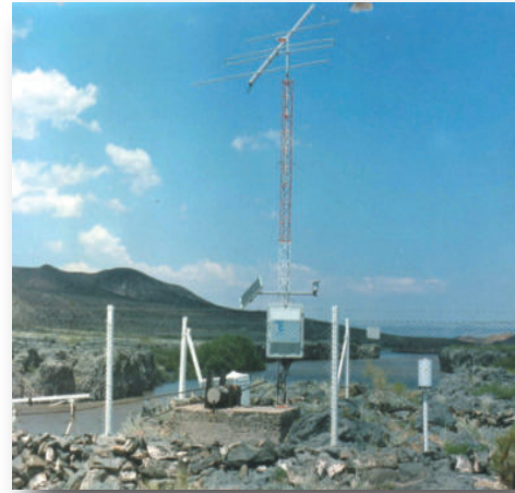
Typical sensors configurable in the Station METEORTEC
