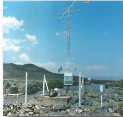
Typical sensors configurable in the Station METEORTEC
