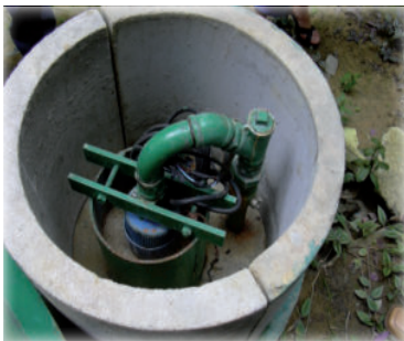
Level control in wells, San Salvador Bay, Brazil
