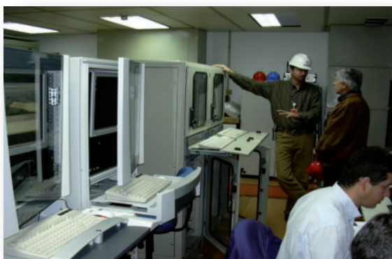
Control room of the ITaipu Dam
