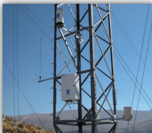
Measurement of snow height and meteorological parameters, Minera Alumbreira, Catamarca, Argentina
