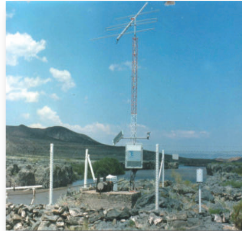
Typical sensors configurable in the Station METEORTEC
