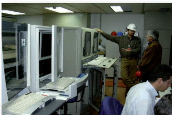
Control room of the ITaipu Dam
